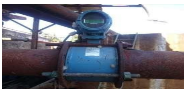
ETP Outlet flow meter
